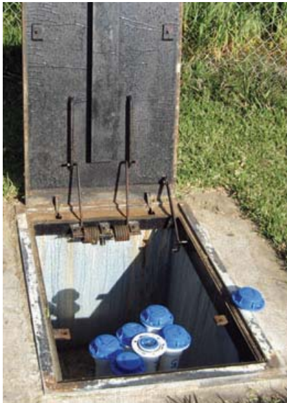
Figure 2. Completed nested monitoring wells for WRD’s monitoring program. Each nested well taps a major aquifer.
